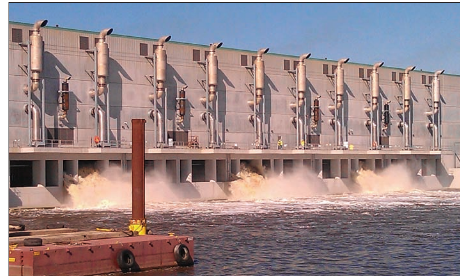
The world's largest drainage pump station keeps water flowing out of town, even when the nation's largest sector gate closes the waterway. PHOTO COURTESY OF WENDI GOLDSMITH
